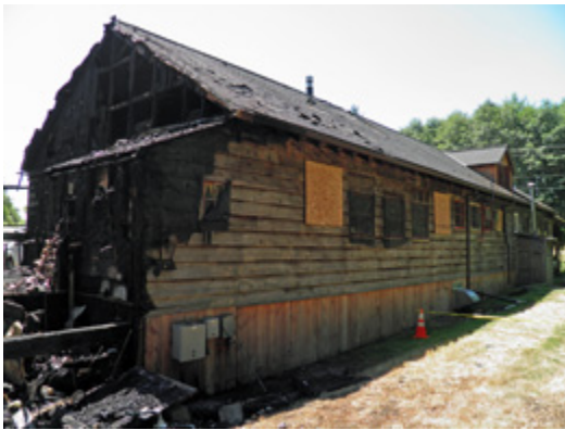
Strawberry Barreling Plant building damaged by fire, Olga, Orcas Island, July 2013
