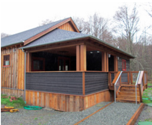
Strawberry Barreling Plant building, restoration work following June 2013 fire, Olga, Orcas Island, March 2015
